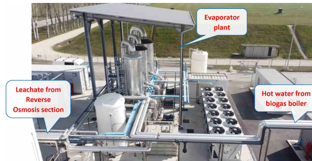
Fig. 1. Evaporation plant: top view [credits: NBT Bulgaria EOOD]
